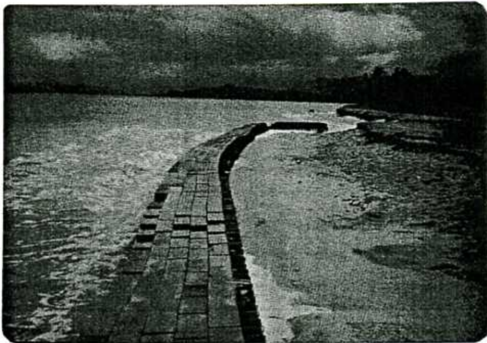
Figure 2-601. Differential settling of individual blocks viewed from structure's midsection, Kualoa, Hawaii, 7 April 1978.
