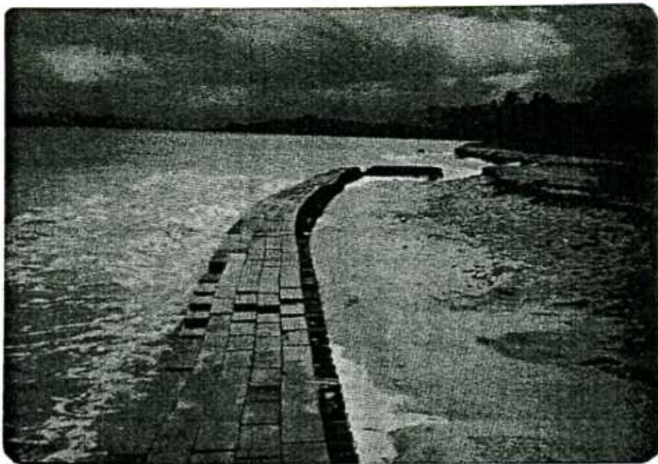
Figure 2-601. Differential settling of individual blocks viewed from structure's midsection, Kualoa, Hawaii, 7 April 1978.
