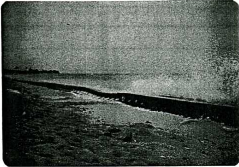
Figure 2-600. Settlement of blocks along midsection, Kualoa, Hawaii, 7 April 1978.
